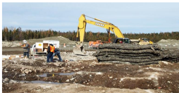
Figure 18 : Mat covering on closest holes to the town
